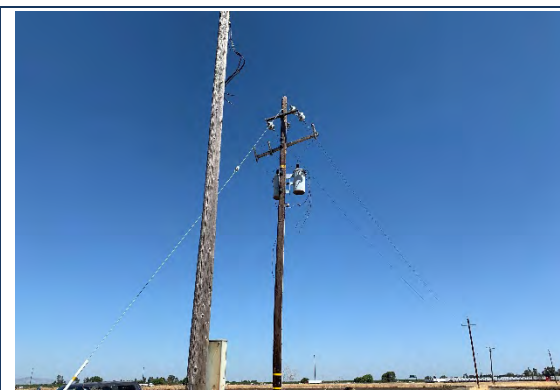
Pole-mounted electrical transformers on northeasterly portion of the property
