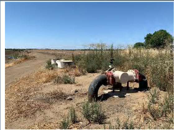
Irrigation water control features on westerly portion of the property
