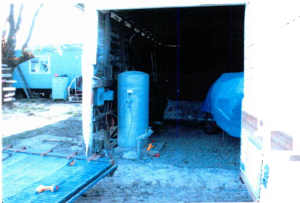
Photograph No. 6. Domestic water well, pump, and small storage tank located at base of building pictured above.
